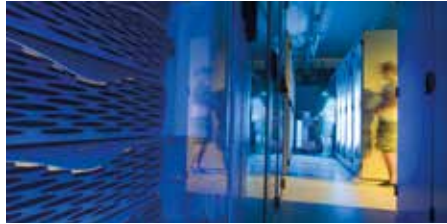
Grid/SCC - A glimpse of the high-performance computing infrastructure of the Grid Steinbuch Centre for Computing Karlsruhe
